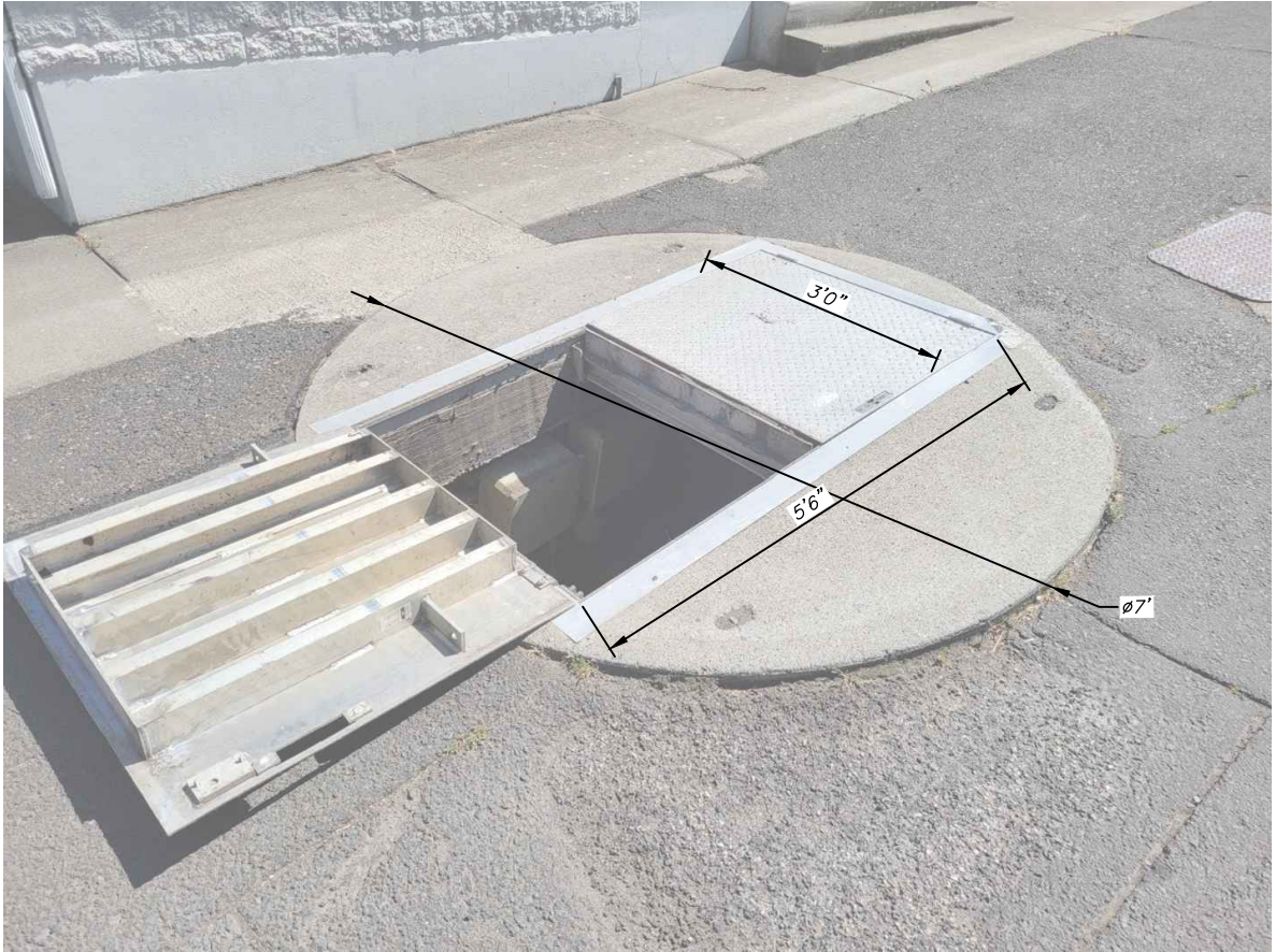
PHOTOGRAPH – HERITAGE PLAZA PUMP STATION EXISTING VAULT HATCH.
