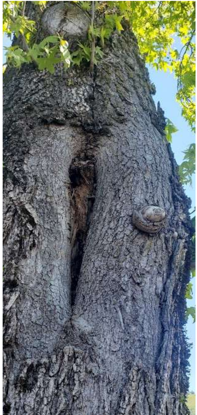
South side limb failure (close up) shows decay/splintered wood indicating prior failure, not pruning wound. Smaller pruning wound above is sealed.
