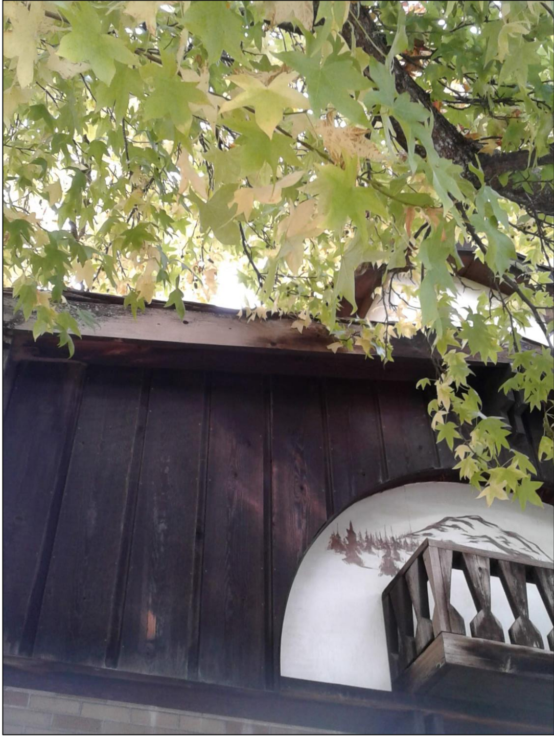
Figure 2: Branches near the roof of the nearby building.
