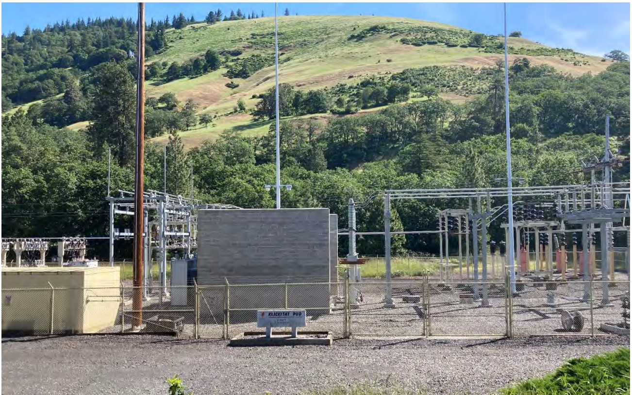
Photo 10. Substation adjoining the property to the west.
