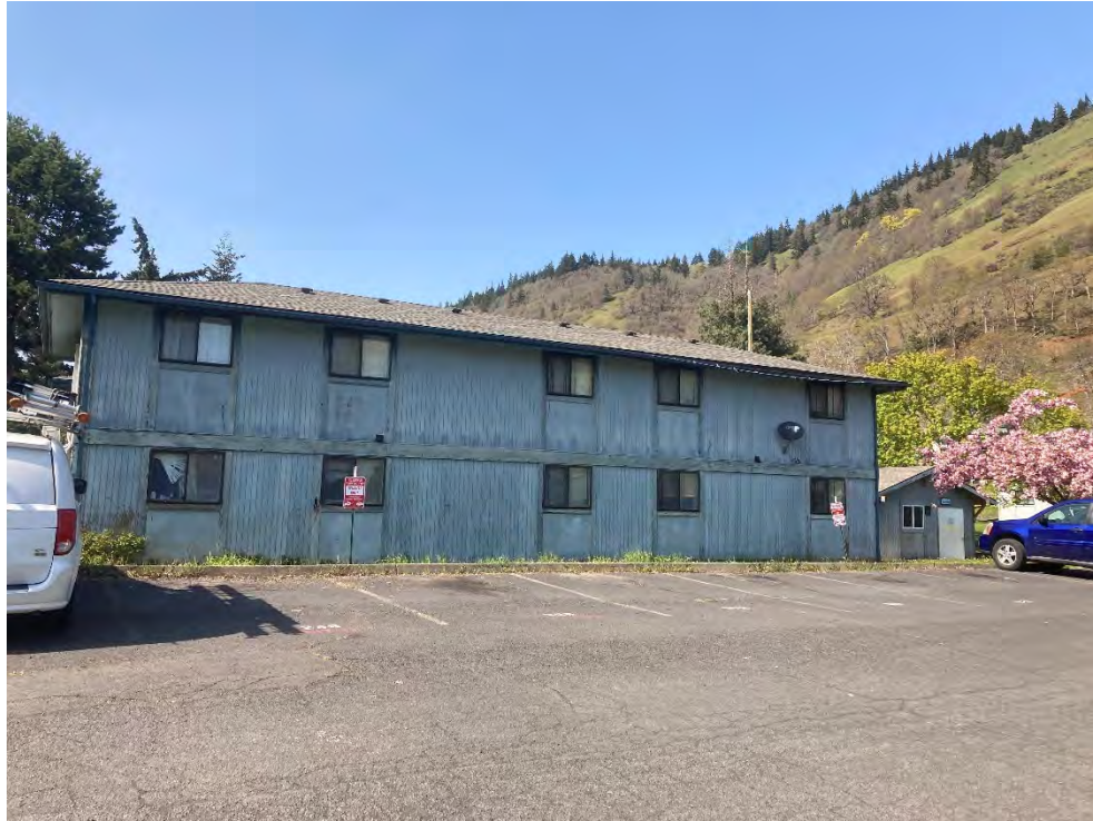
Photo 1. Parking area and two-story residential building at the east end of the complex, from the Southeast.
