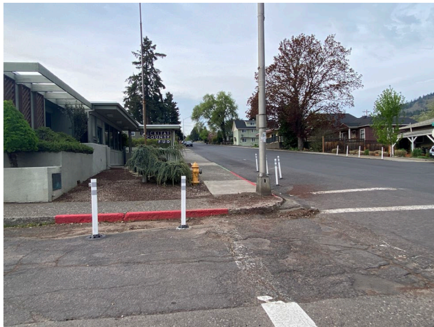
Some streets that do have sidewalks do not have curb ramps at corners, even where marked crosswalks are striped. Maintenance of existing roadways remains a priority for the City.
