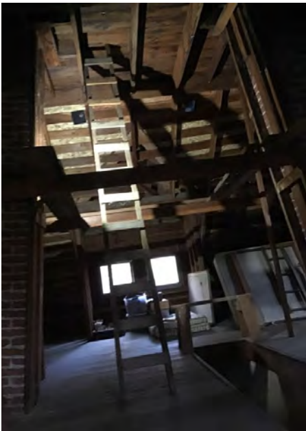
Unsafe ladder access to flat portion fo the roof- excluded- not inspected.
