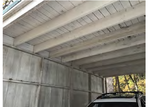
No diagonal support work and or metal supports
