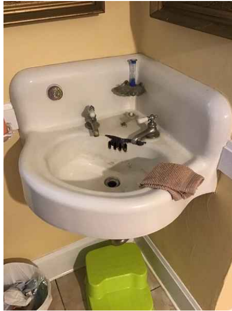
Older corner sink with damage (chipped) noted. No shut off valves noted below the sink.
