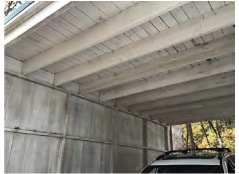
No diagonal support work and or metal supports
