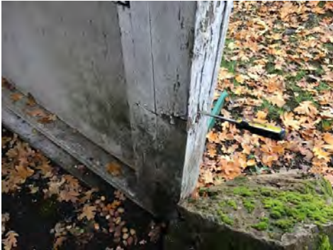
Southwest corner Wood Decay
