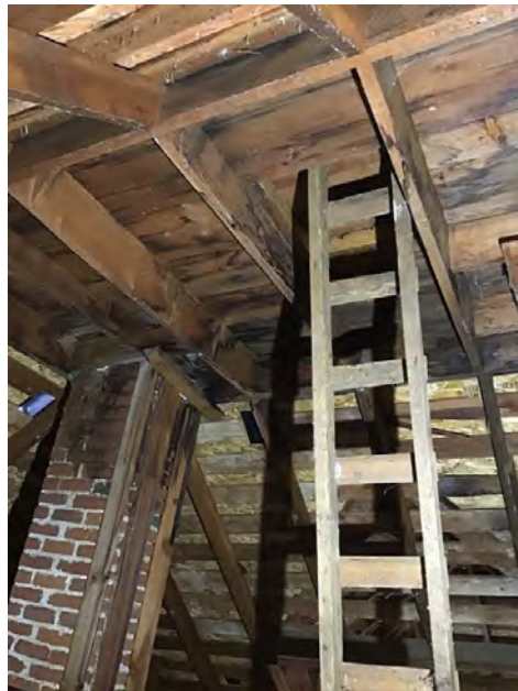
Indications of past leaking noted- None at the time of the inspection.
