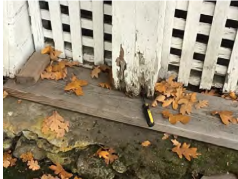
Northeast Side- Post floating and damaged
