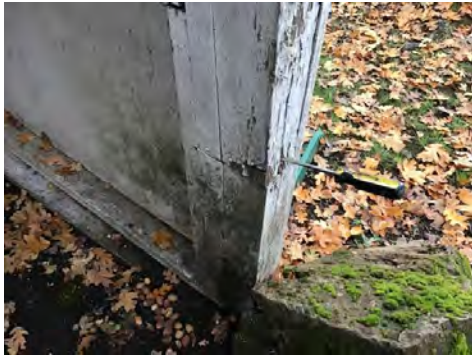
Southwest corner Wood Decay
