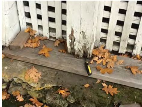
Northeast Side- Post floating and damaged
