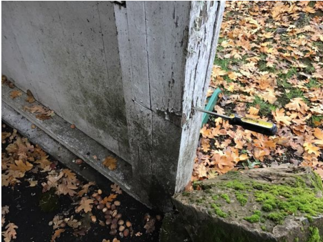
Southwest corner Wood Decay
