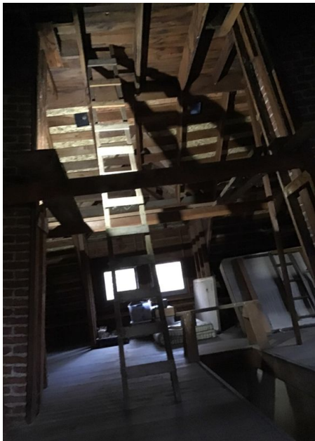
Unsafe ladder access to flat portion fo the roof- excluded- not inspected.
