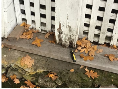
Northeast Side- Post floating and damaged
