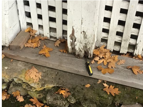
Northeast Side- Post floating and damaged
