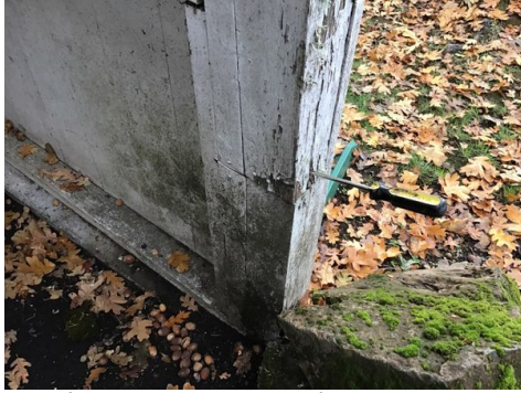
Southwest corner Wood Decay
